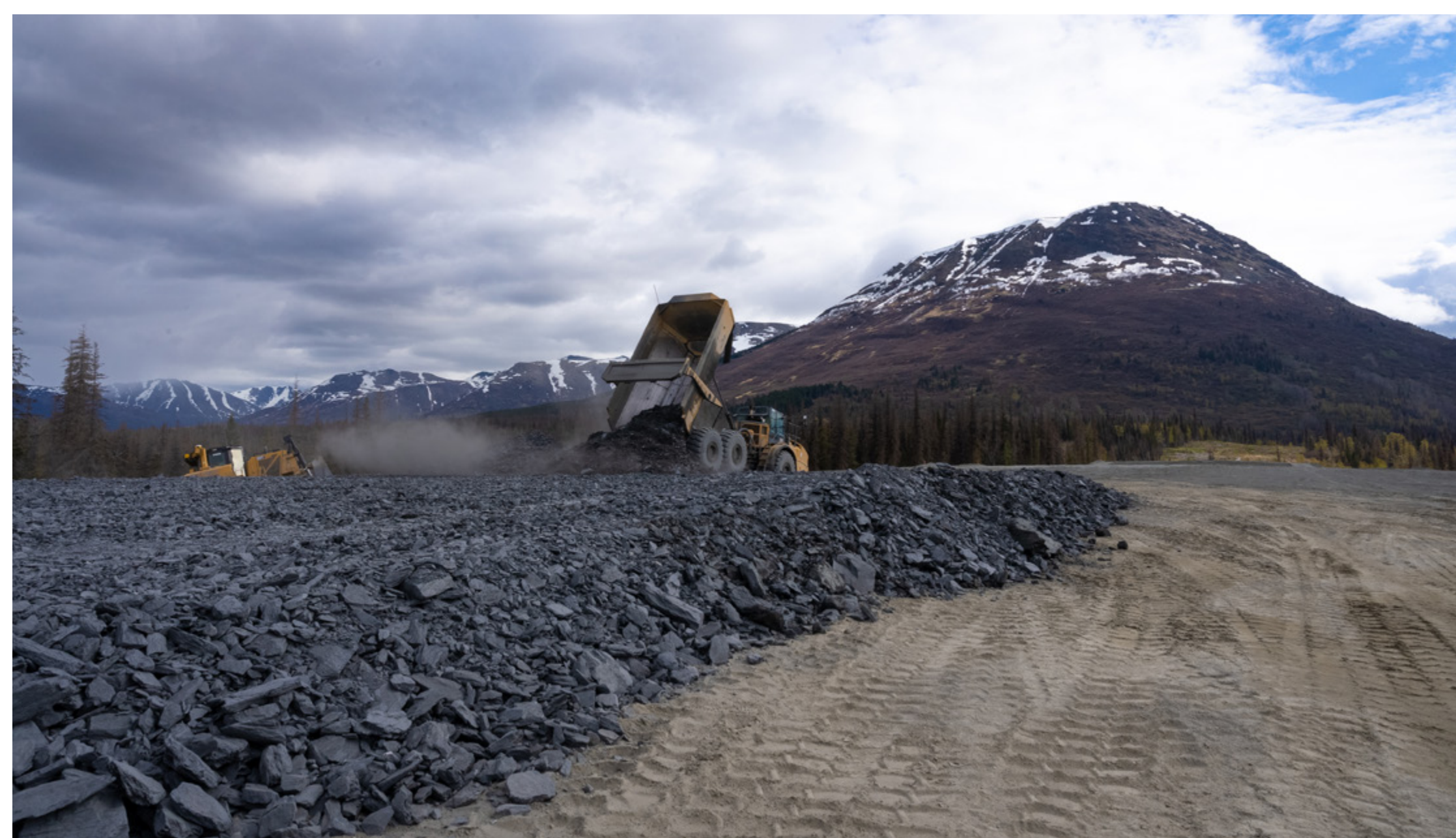
Material from Phase 1B will be Trucked to Build up Final Road
