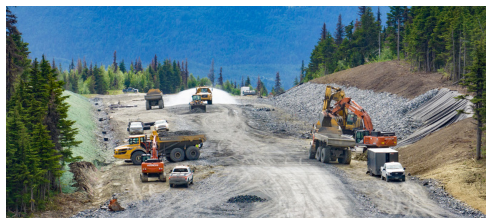
Phase 4: Installation of an underdrain system on the west side of Juneau Creek
